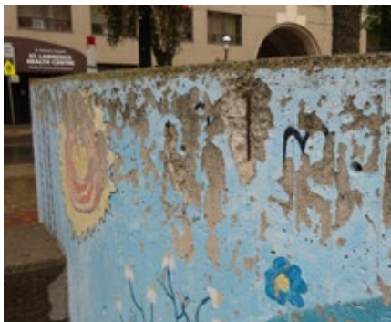
The park is showing its age Many features are original (40 years old) and need repair or replacement.
